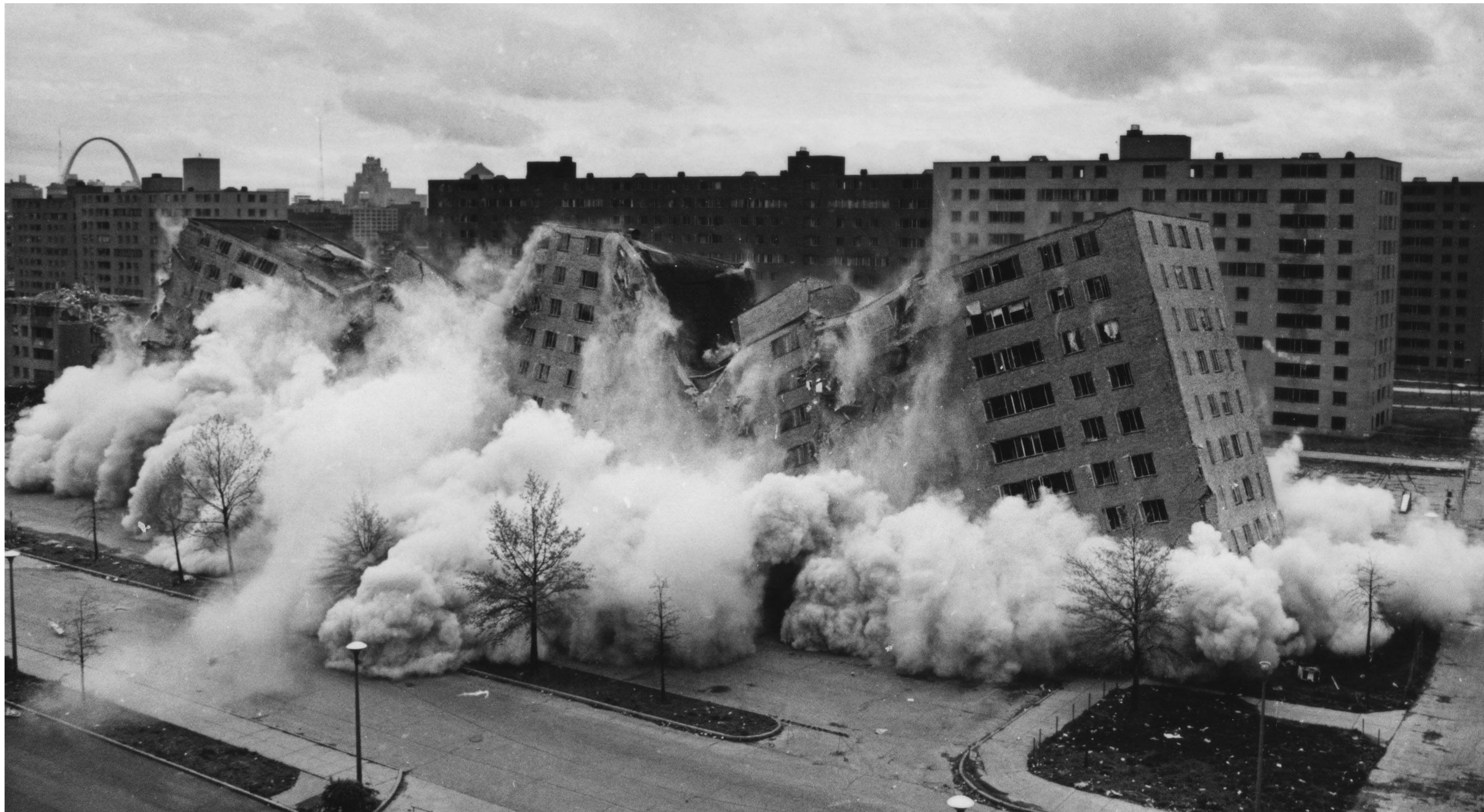
The demolition of 3 of Pruitt Igoe's 33 total building on June 15th, 1972. Demolition was complete by 1976. Photo Courtesy of PD&R Edge Magazine
